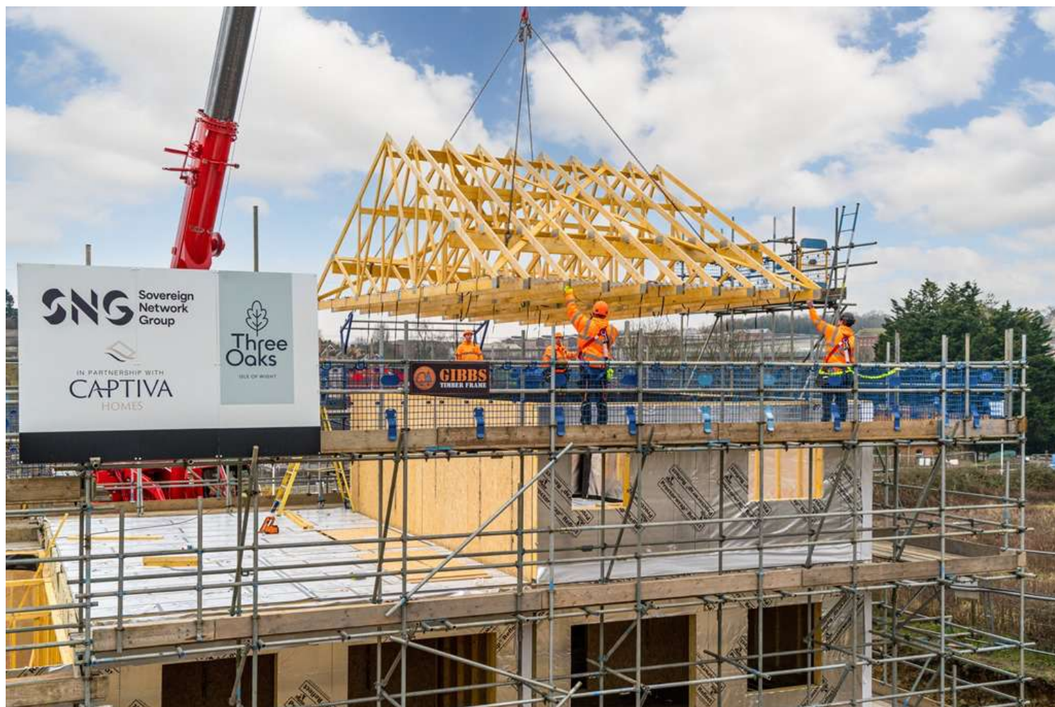
Above: Gibbs Timber Frame erected three houses in a day at Newport's Three Oaks development
